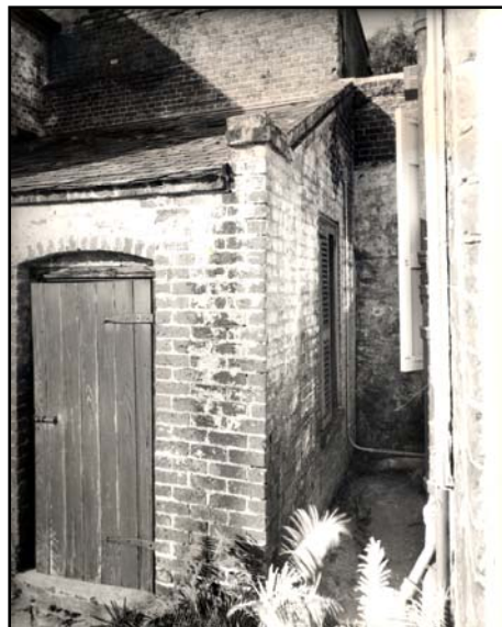
Figure 14: the pantry and cistern, added between the kitchen and main house in the 19 th century.
